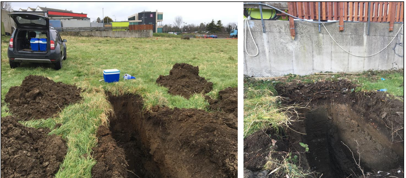
Plate 1 Petrol Station and area of contamination). Plate 2 TP18-11 at boundary of petrol station. (Looking North)
